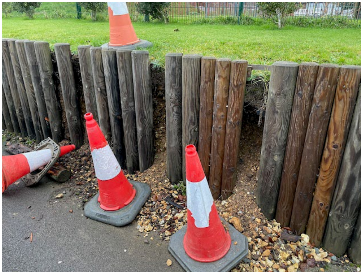
Figure 1 – Rotten/rotting wooden retaining posts
