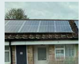
Photovoltaic Solar Panels
