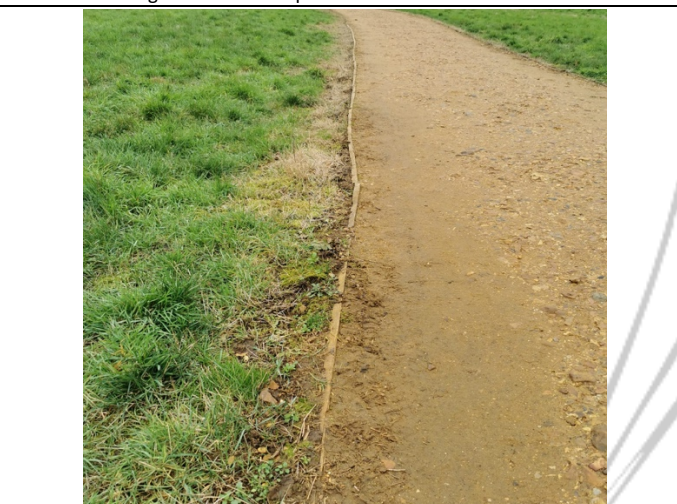
Plate 18 – Footpath edging in need of repair
