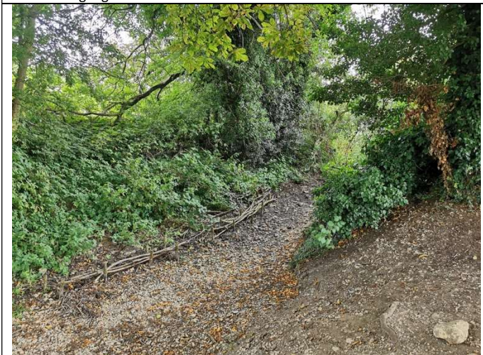
Plate 3 – Berm in need of repair upstream of Lenten Street Bridge
