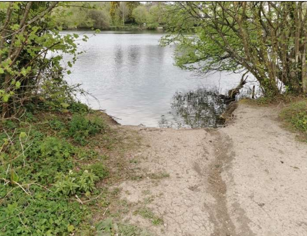
Plate 17 – Typical area of bank erosion to be repaired
