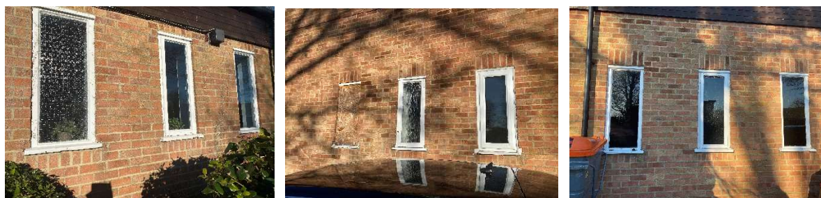
(An example of the remaining windows that need replacing)
